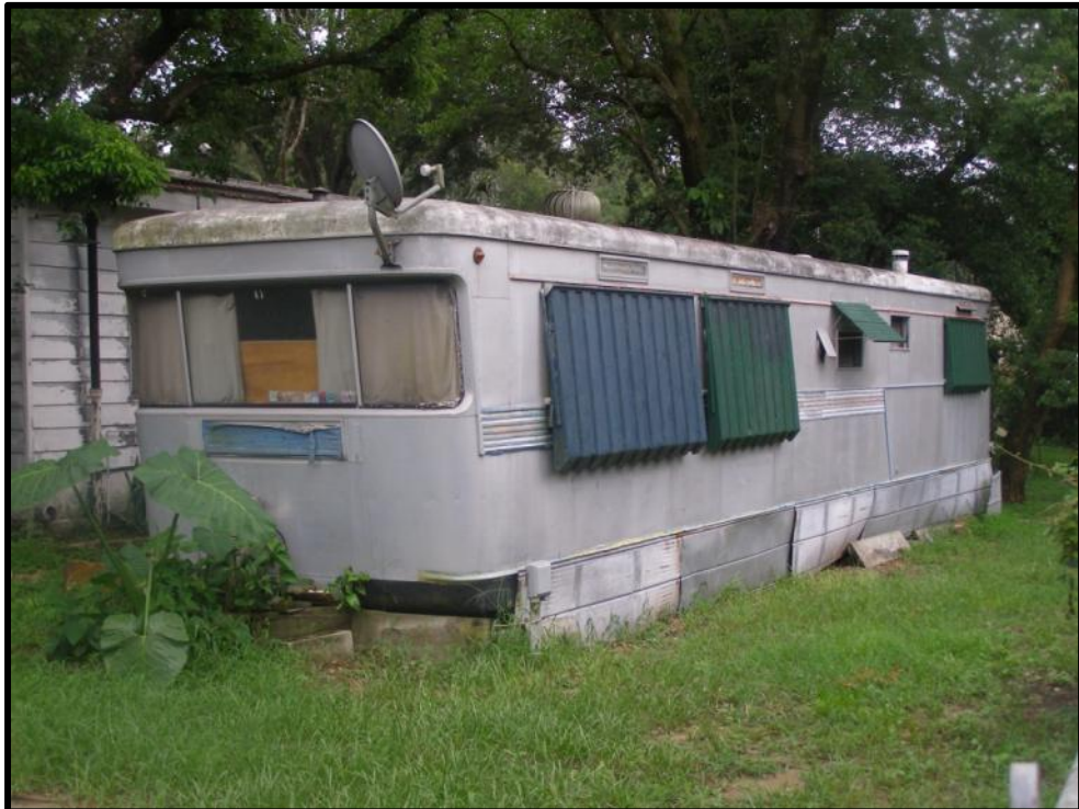
Photo 6-16. The north and west elevations of the mobile home at 102B Sharewood Drive (8HI11969).
