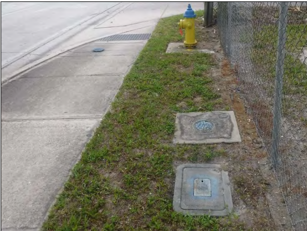
Figure 10-15 Representative View of Indicators of Underground Utilities and Hardscape Preventing Testing Along US 41, Facing North Along US 41
