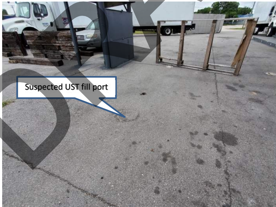
Site 67 – Avengers Auto Body/DMD Motors (former CSD Truck Repairs) West-central area looking south
