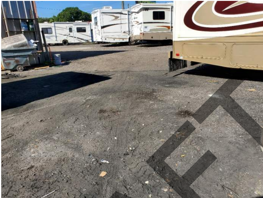
Site 65 –RV Depot Stained soils near northwest corner of building, looking southwest
