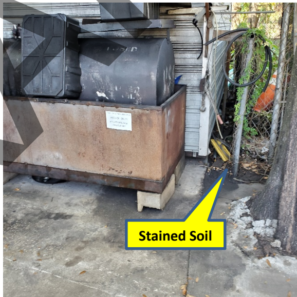
POND 3B – Cabellero Auto (West parcel) South of waste oil AST looking north
